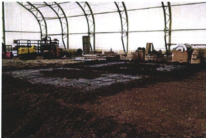
Figure 10 – Completed test pad covered with a plastic tarp in order to maintain the original water content at which the BAS was placed and compacted.
